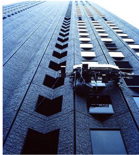
Fig. 6. Single-task construction robot applied by the company Taisei to automatically coat and paint the façade of a high-rise building.
